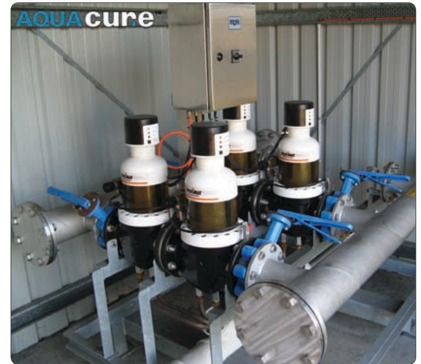
Skid mounted system with four DN80 units
